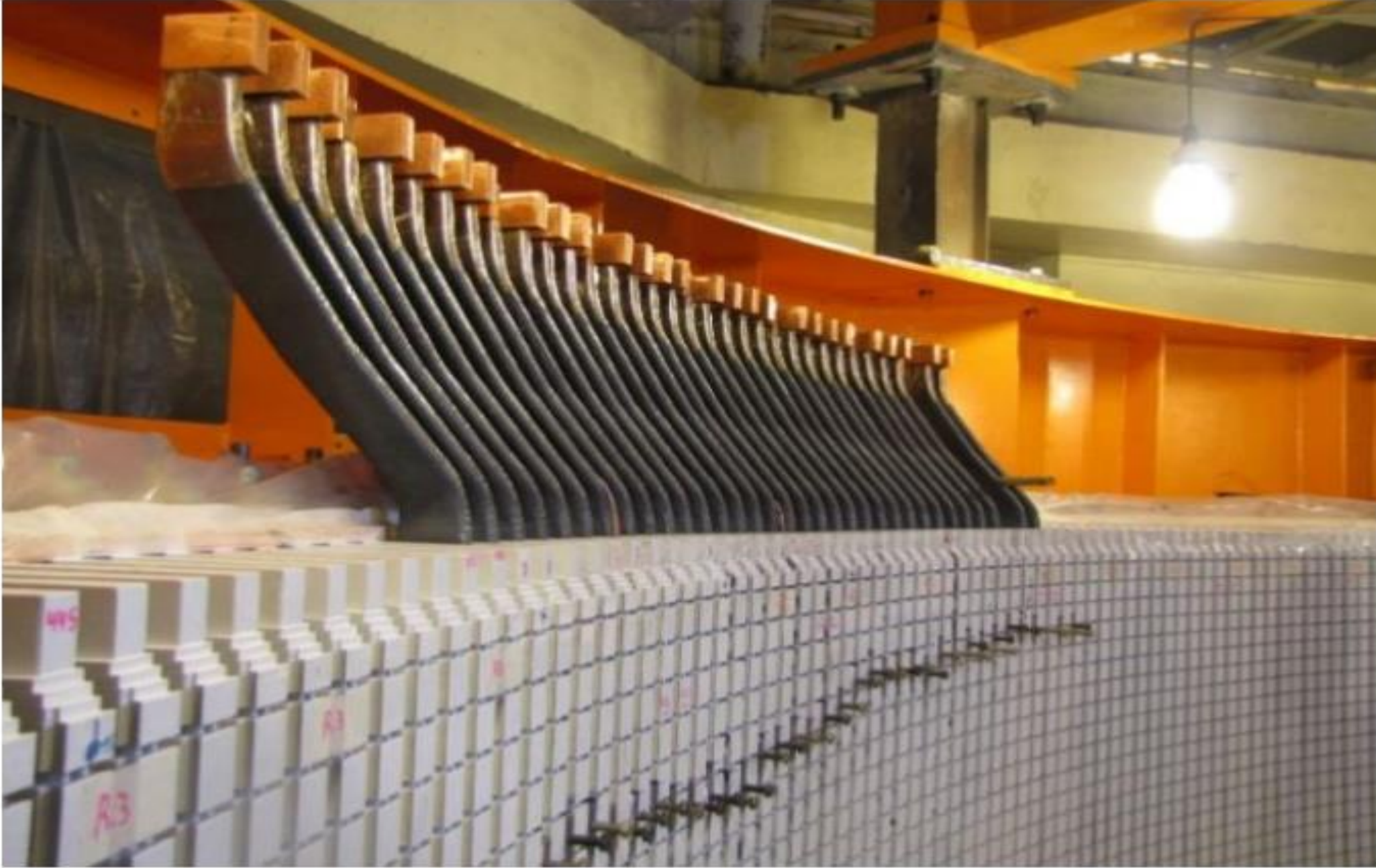
Part of stator winding of a 160 MW, 32-pole hydro generator at the Samira Power Plant, located in Iran.
